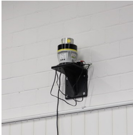
Figure 2.1: iGPS transmitter (fixed)
